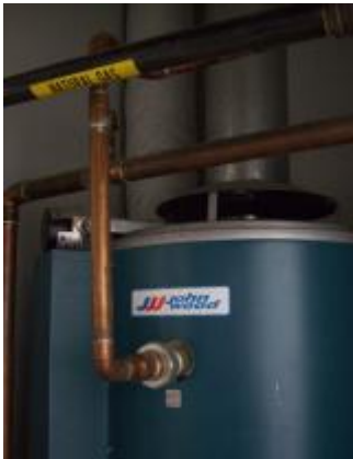
Insulated water pipes, an example of low lying fruit.
