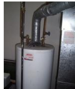
Insulated water pipes, an example of low lying fruit.
