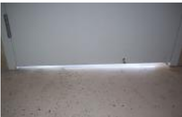
Opportunity for weather stripping to minimize heat loss.
